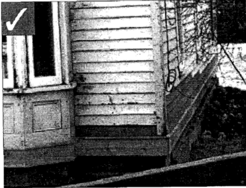
Repair wood features by patching or piecing-in new wood elements that match the original.
