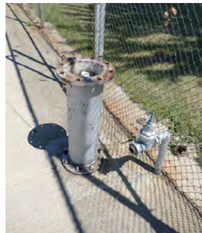
Unuseable drinking fountain
