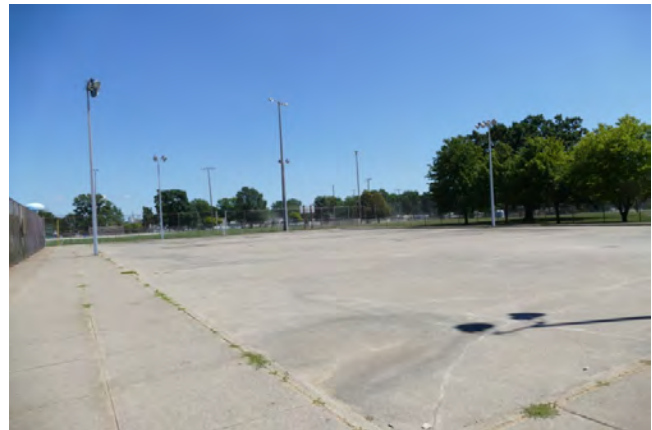
Cement surface with no function
